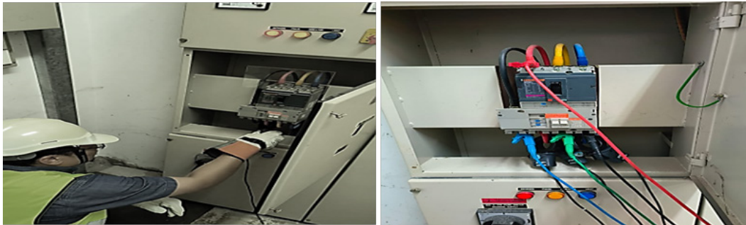
Figure 2: Electricity Supply System Electrical Distribution Box
